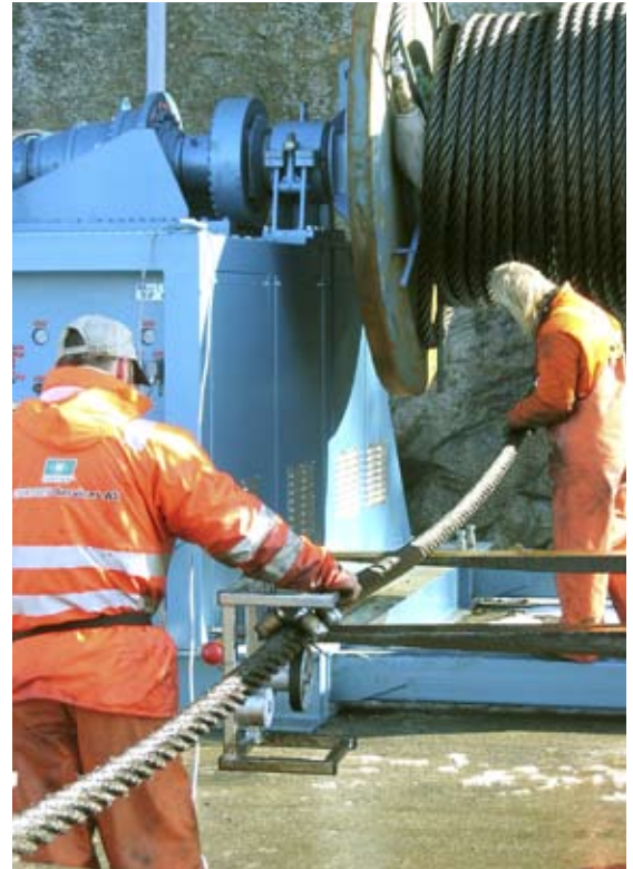
Our riggers at work on the winding machine at our deepwater quay in Bergen.
